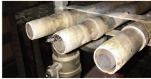
Figure 5. Carbon build-up on natural gas nozzle tip of HeatOx burner
